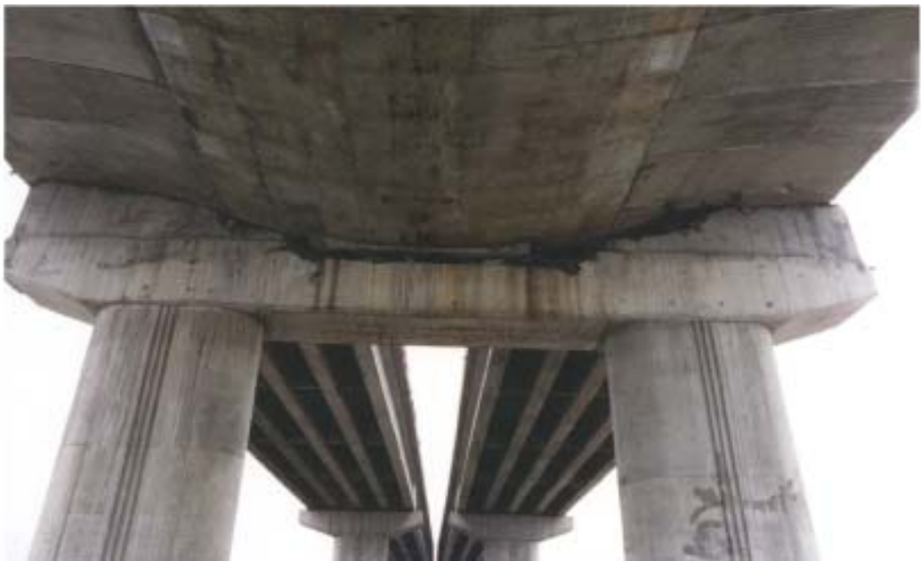
FIGURE 30.45 Damage at end-supports to Ji Lu cable-stayed bridge.
