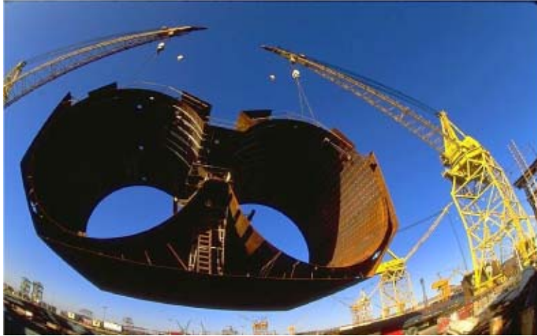
FIGURE 15B.3 Steel immersed tunnel: Ted Williams Tunnel, Boston, MA. (© David Sailors, 1993. With permission.)
