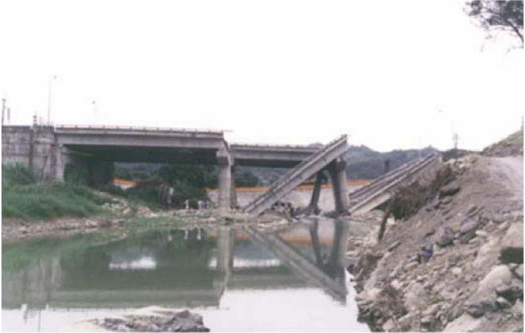
FIGURE 30.19 Collapse of Tsu Wei Bridge due to landslide during the Ji Ji, Taiwan earthquake.
