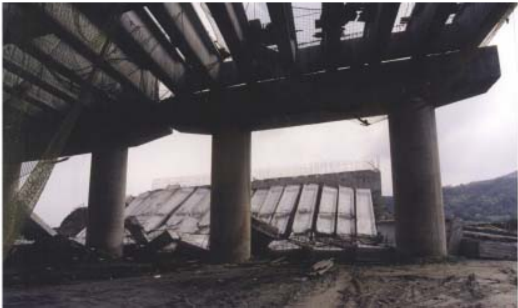
FIGURE 30.63 Precast, prestressed “I” girders during construction of new expressway in Taiwan that collapsed during the 1999 Ji Ji, Taiwan earthquake.
