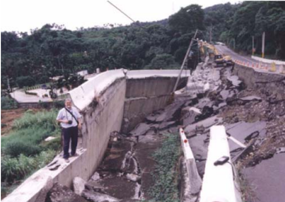
FIGURE 30.13 Gravity retaining wall pushed outward by landslide.
