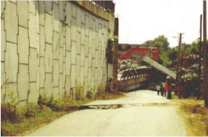
FIGURE 30.73 Mechanically stabilized earth (MSE) wall continues to support the embankment behind the collapsed Arifiye Overcrossing after the 1999 Kocaeli, Turkey, earthquake.
