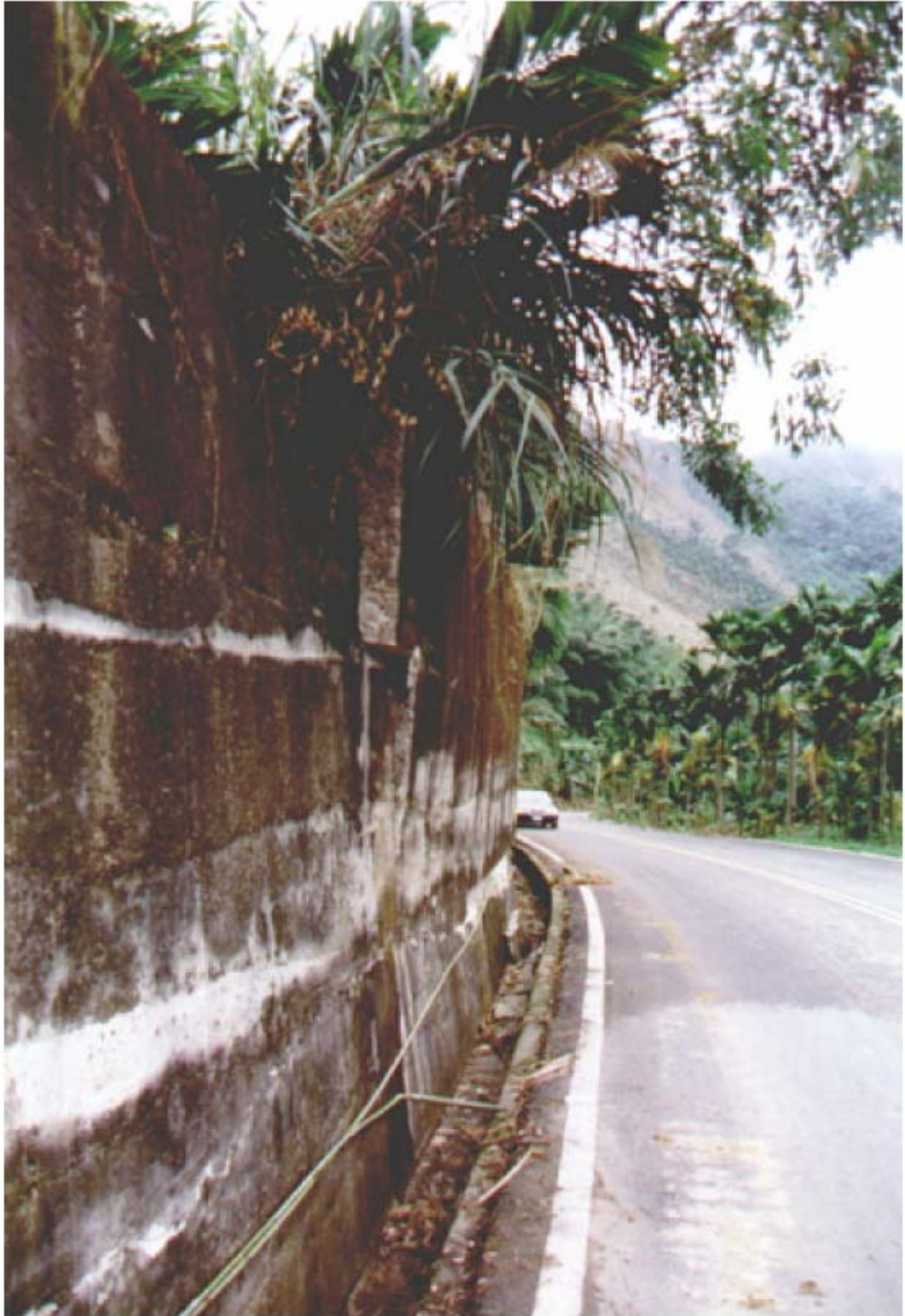
FIGURE 30.14 Gravity retaining wall with shear damage from landslide.
