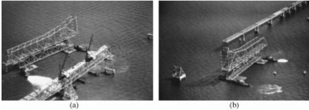
FIGURE 20.30: Floating-in erection of a truss span, first Chesapeake Bay Bridge, Maryland, 1951. Erected 300-ft (91-m) deck-truss spans form erection dock, providing a work platform for two derrick travelers. A permanent deck-truss span serves as a falsework truss supported on barges and is shown carrying the 470-ft (143-m) anchor arm of the through-cantilever truss. This span is floated to its permanent position, then landed onto its piers by ballasting the barges. (a) Float leaves erection dock, and (b) float arrives at permanent position. (Courtesy of Bethlehem Steel Corporation.)
