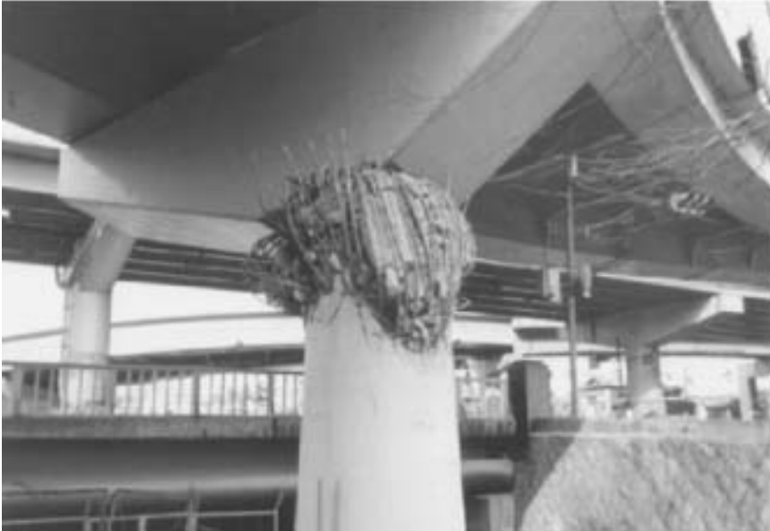
FIGURE 30.46 Column damage to the Minatogawa Interchange during the Kobe earthquake.
