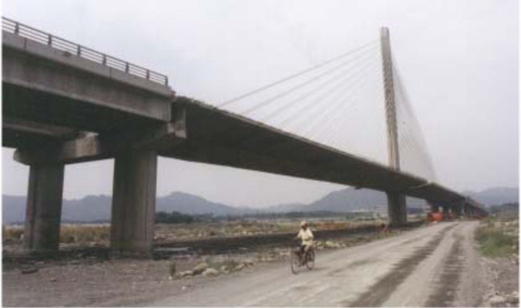
FIGURE 30.44 The Ji Lu cable-stayed bridge after the 1999 Taiwan earthquake.
