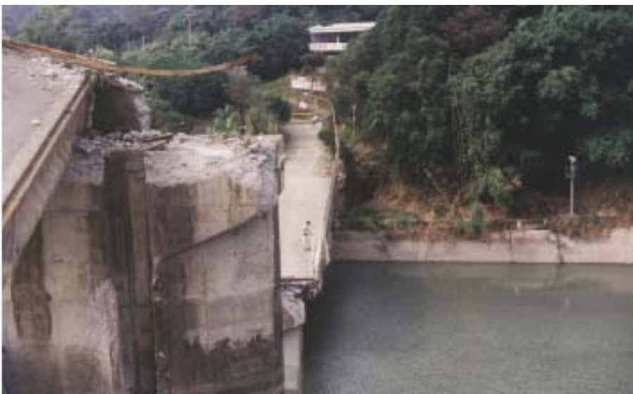
FIGURE 30.65 North end of Shih Kang Dam after the Ji Ji, Taiwan earthquake.
