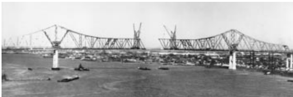
FIGURE 20.34: Greater New Orleans cantilever bridge, Louisiana, 1957. Tall double-boom deck travelers started at ends of main bridge and erected anchor spans on falsework, then the 1575-ft (480-m) main span by cantilevering to midspan. (Courtesy of Bethlehem Steel Corporation.)
