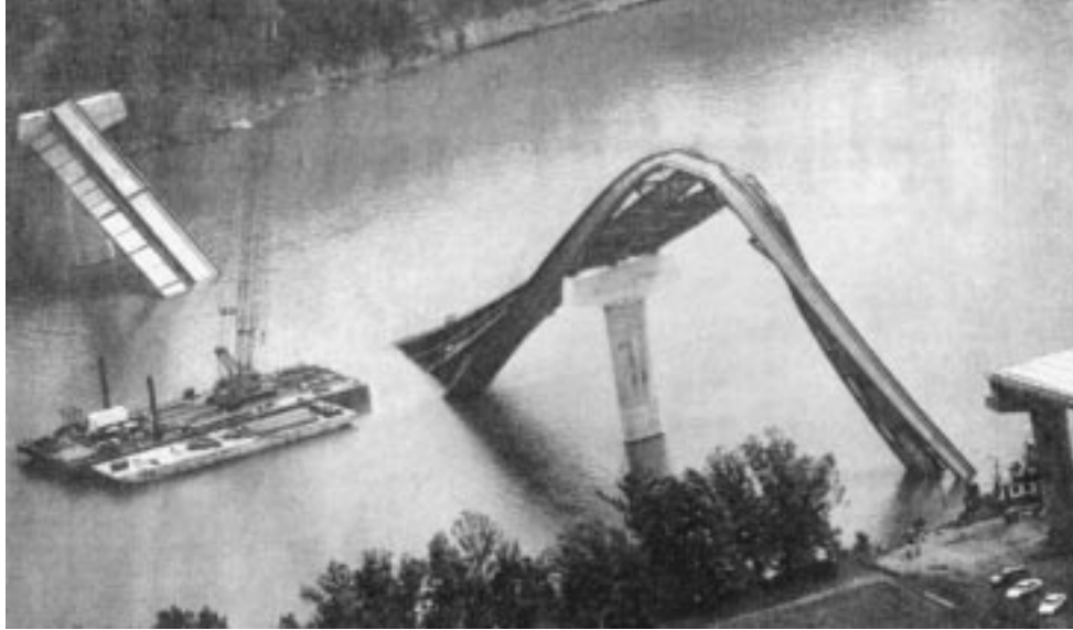
FIGURE 20.1: Failure of a steel girder bridge during erection, 1995. Steel bridge failures such as this one invite suspicion that the construction engineering aspects were not properly attended to.
