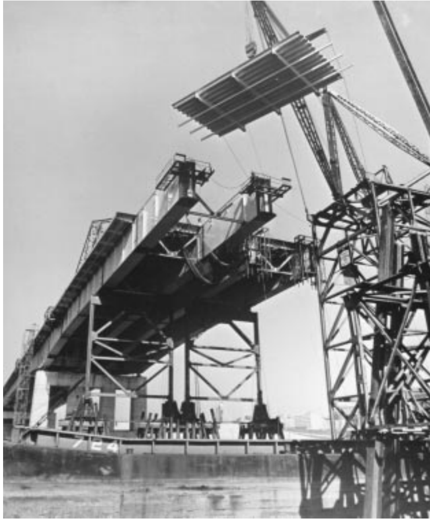
FIGURE 20.36: Erecting orthotropic-plate decking panel, Poplar Street Bridge, St. Louis, Mo., 1967. A five-span, 2165-ft (660-m) continuous box-girder bridge, main span 600 ft (183 m). Projecting box ribs are 5\text{-}1/2 \times 17 ft ( 1.7 \times 5.2 m) in cross-section, and decking section is 27 \times 50 ft ( 8.2 \times 15.2 m). Decking sections were field welded, while all other connections were field bolted. Box girders are cantilevered to falsework bents using overhead “positioning travelers” (triangular structure just visible above deck at left) for intermediate support. (Courtesy of Bethlehem Steel Corporation.)
