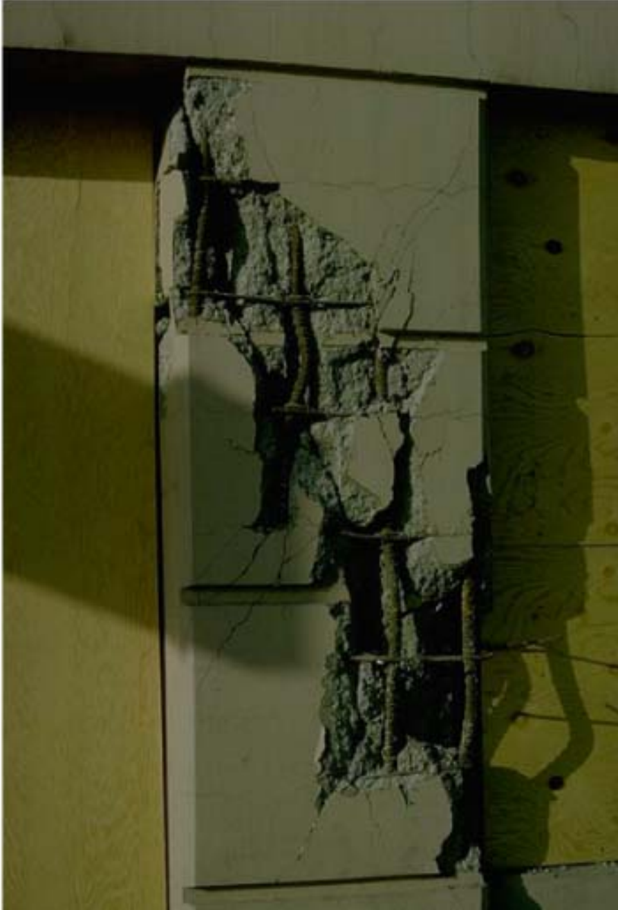
FIGURE 30.50 Damage to the south side of Mt. McKinley Apartments. (Photograph by Karl Steinbrugge and courtesy of the Steinbrugge Collection, Earthquake Engineering Research Center, University of California, Berkeley.)
