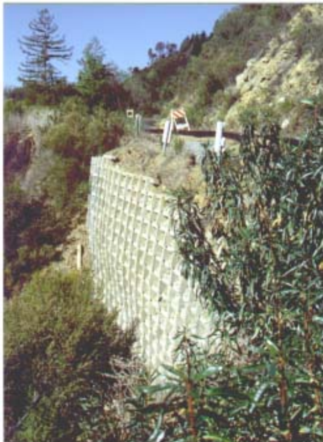
FIGURE 30.74 Crib wall continues to support steeply sloping soil in Santa Cruz after the 1989 Loma Prieta earthquake. (Courtesy of the Earthquake Engineering Research Institute; photograph by Marshall Lew [1a].)
