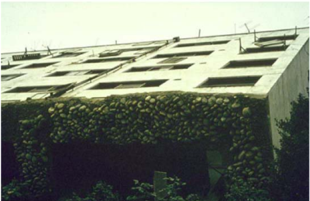
FIGURE 30.5 Liquefaction-caused building failure in Niigata, Japan. (Photograph by Joseph Penzien and courtesy of Steinbrugge Collection, Earthquake Engineering Research Center, University of California, Berkeley.)
