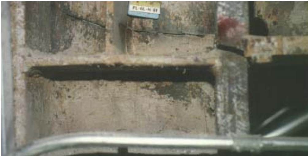
FIGURE 30.60 Steel moment-resisting frame connection after the 1994 Northridge earthquake. (From EQE International, Inc., Steel's performance in the Northridge earthquake , EQE International Fall Review , p. 1, 1994. With permission.)
