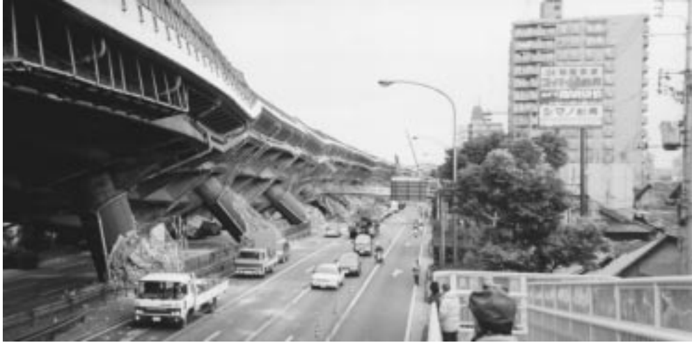
FIGURE 16.5: Collapsed Hanshin Expressway following the 1995 Kobe earthquake in Japan. (Photo by Mark Yashinsky. With permission.)
