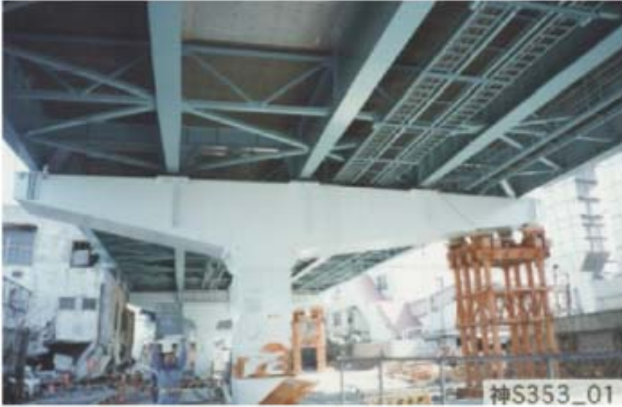
FIGURE 30.68 Collapsed building leaning against the Kobe Route 3 Expressway. (Courtesy of Hanshin Expressway Public Corporation.)
