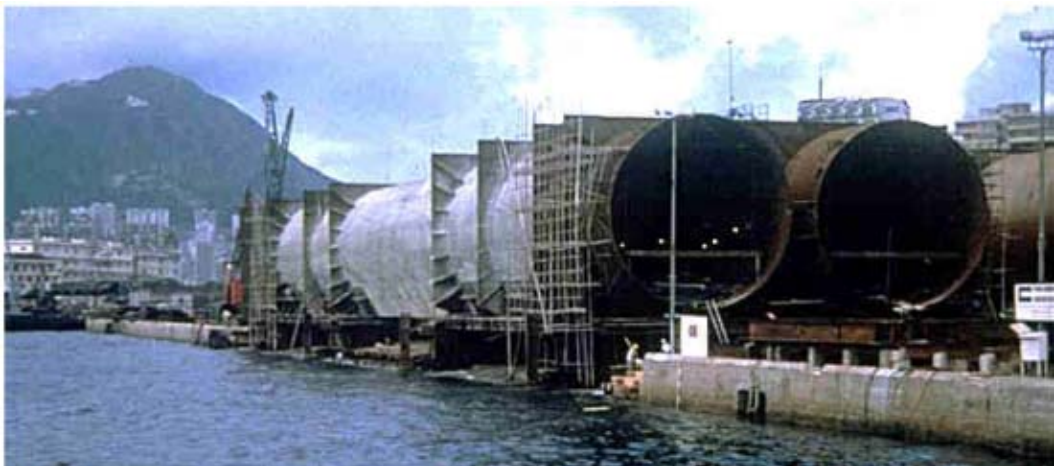
FIGURE 15B.4 Steel immersed tunnel: Cross Harbour Tunnel, Hong Kong. (© Parsons Brinckerhoff, Inc., 1971. With permission.)
