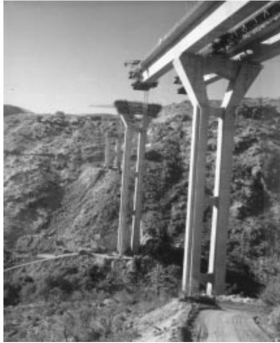
FIGURE 10.16 Pine Valley Bridge, California. Construction state. (From California Department of Transportation. With permission.)
