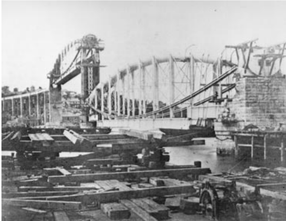
FIGURE 20.14: Royal Albert Bridge across River Tamar, Saltash, England, 1857. The two 455-ft (139-m) main spans, each weighing 1060 tons, were constructed on shore, floated out on pairs of barges, and hoisted about 100 ft (30 m) to their final position using hydraulic jacks. Pier masonry was built up after each 3-ft (1-m) lift.
