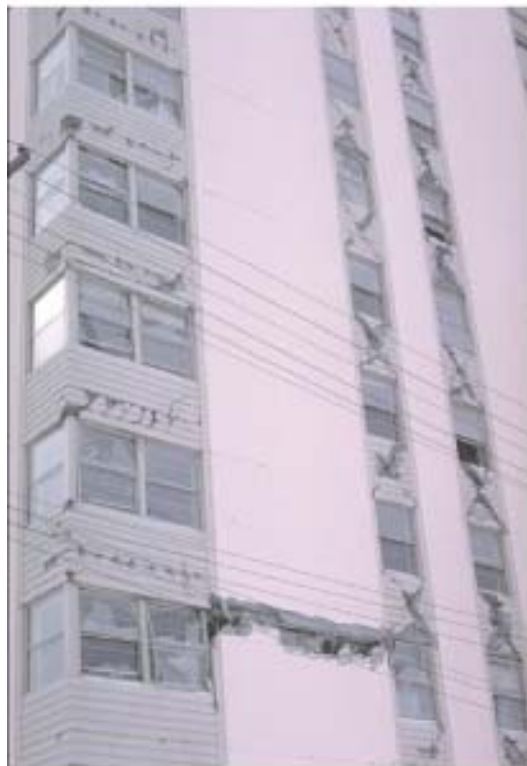
FIGURE 30.49 Damage to north side of Mt. McKinley Apartments. (Photograph by Karl Steinbrugge and courtesy of the Steinbrugge Collection, Earthquake Engineering Research Center, University of California, Berkeley.)
