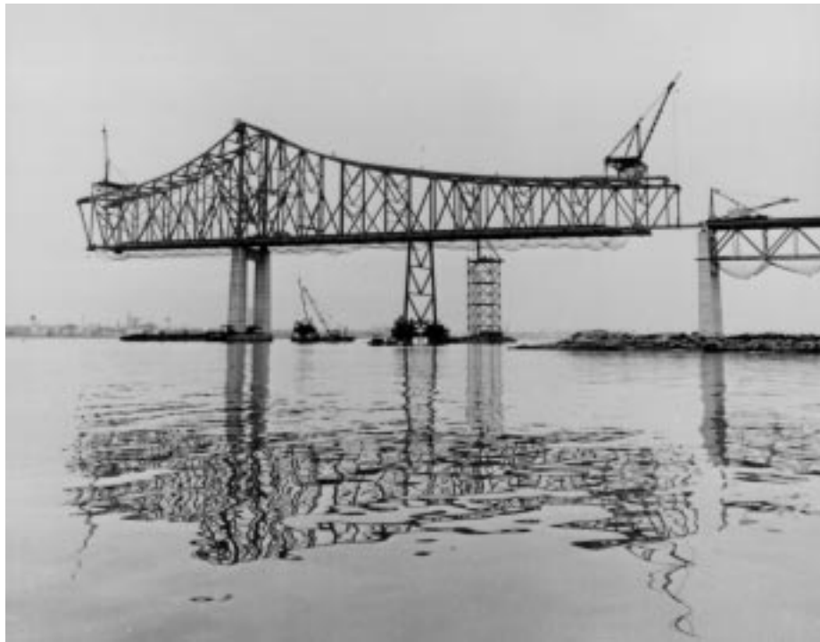
FIGURE 20.44: Closure of east side span, Commodore John Barry cantilever truss bridge, Chester, Pa., 1973. A high-tower derrick boat (in background) started erection of trusses at both main piers, supported on falsework; then erected top-chord travelers for main and side spans. The sidespan traveler carried steelwork erection to closure, as shown, and the falsework bent was then removed. The mainspan traveler then cantilevered the steelwork (without falsework) to midspan, concurrently with erection by the west-half mainspan traveler, and the trusses were closed at midspan. Commodore Barry has a 1644-ft (501-m) main span, the longest cantilever span in the U.S., and 822-ft (251-m) side spans. (Courtesy of Bethlehem Steel Corporation.)
