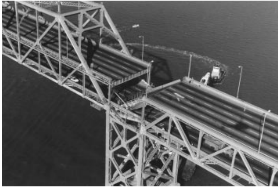
FIGURE 16.2: Aerial view of collapsed upper and lower decks of the San Francisco-Oakland Bay Bridge (I-80) following the 1989 Loma Prieta earthquake in California. (Photo by California Department of Transportation. With permission.)
