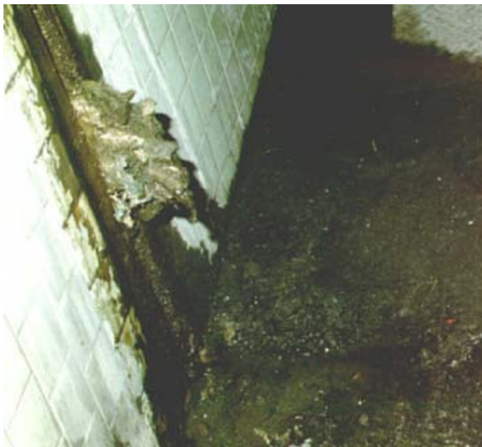
FIGURE 30.11 Liquefaction-induced damage to Webster Street Tube tunnel.
