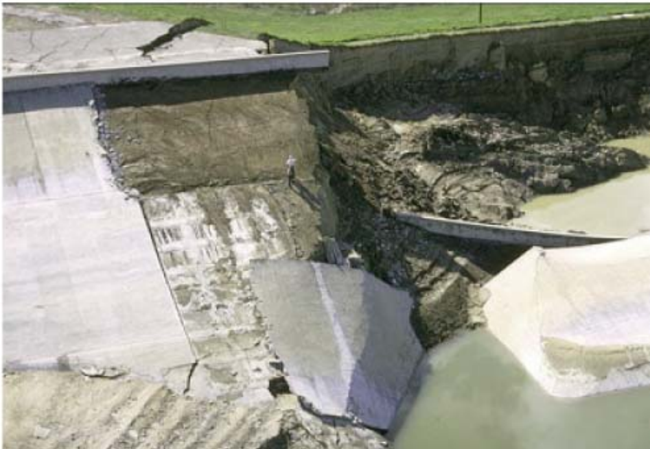
FIGURE 30.22 Closer view of damage to the Lower San Fernando Dam. (Courtesy of Steinbrugge Collection, Earthquake Engineering Research Center, University of California, Berkeley.)
