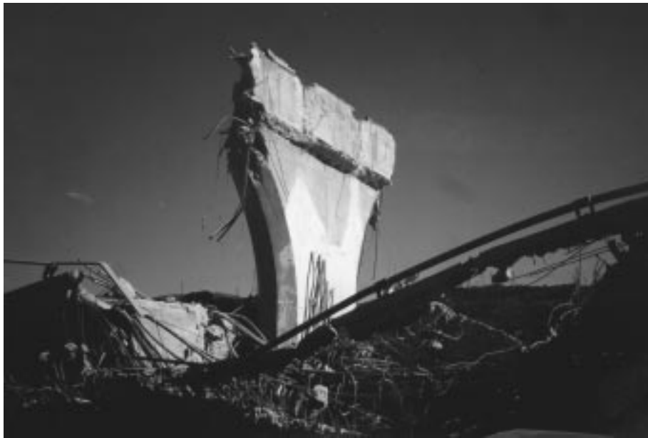
FIGURE 16.4: Collapsed SR-14/I-5 south connector overhead following the 1994 Northridge earthquake in California. (Photo by James MacIntyre. With permission.)
