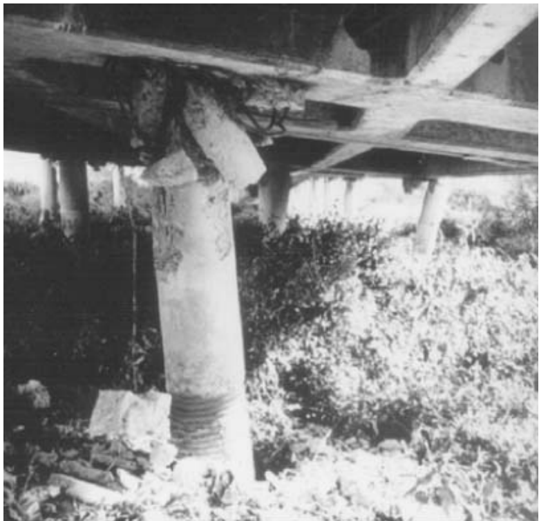
FIGURE 30.25 Broken piles under the bridge.
