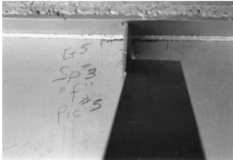
FIGURE 24.9: Typical distortion-induced cracking in the web gap of an attachment plate.
