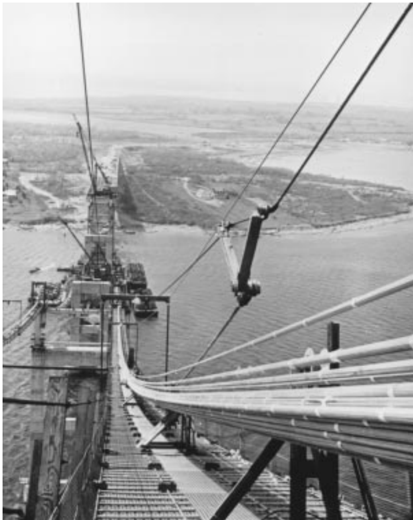
Figure 20.37a Aerial tramway tows PWS from west anchorage up side span, then on across other spans to east anchorage. Strands are about 1-3/4 in. (44 mm) in diameter.
