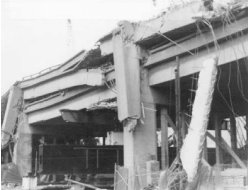
FIGURE 30.28 Damage to Cypress Street viaduct.
