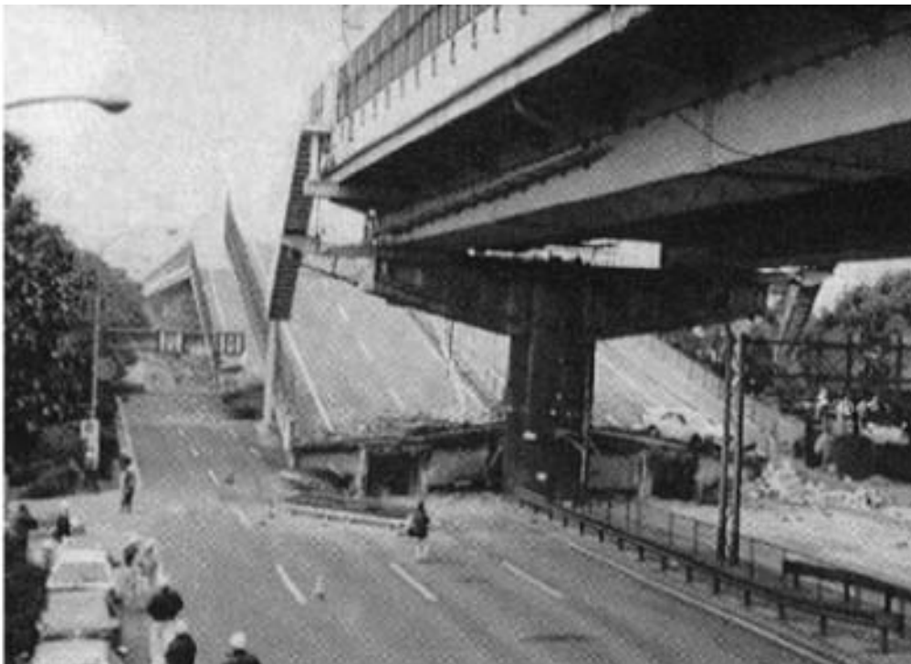
FIGURE 30.56 Superstructure collapse at Spans 40 and 41 on Kobe Route 3.
