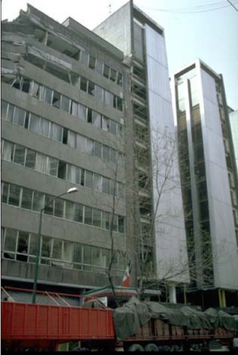
FIGURE 30.31 Damaged 10-story building between the Plaza de la Constitution and Zona Rosa in Mexico City. (Photograph by Karl Steinbrugge and courtesy of the Steinbrugge Collection, Earthquake Engineering Research Center, University of California, Berkeley.)
