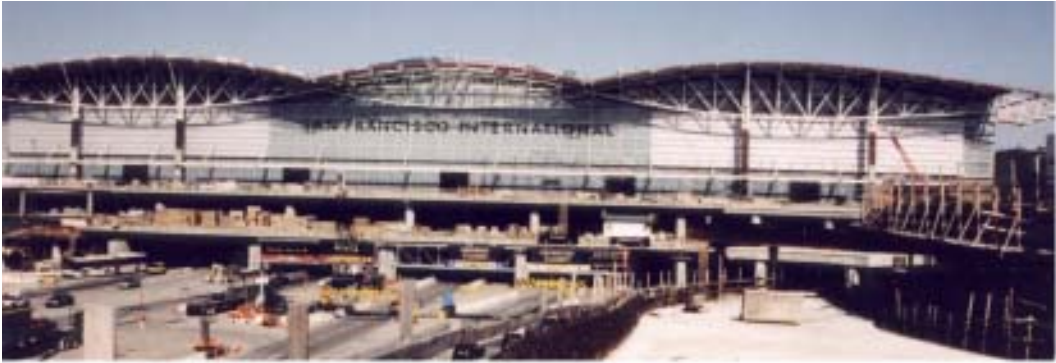
FIGURE 30.77 Construction of the new San Francisco Airport International Terminal. (Courtesy of Earthquake Protection Systems, Inc.)
