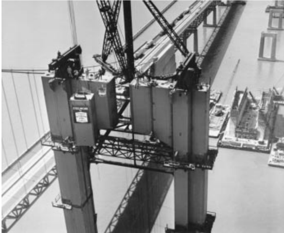
FIGURE 20.35: Tower erection, second Delaware Memorial Bridge, Wilmington, Del., 1966. The tower erection traveler has reached the topmost erecting position and swings into place the 23-ton closing top-strut section. The tower legs were jacked apart about 2 in. (50 mm) to provide entering clearance. The traveler jumping beams are in the topmost working position, above the cable saddles. The tower steelwork is about 418 ft (127 m) high. Cable anchorage pier is under construction at right. First Delaware Memorial Bridge (1951) is at left. The main span of both bridges is 2150 ft (655 m). (Courtesy of Bethlehem Steel Corporation.)
