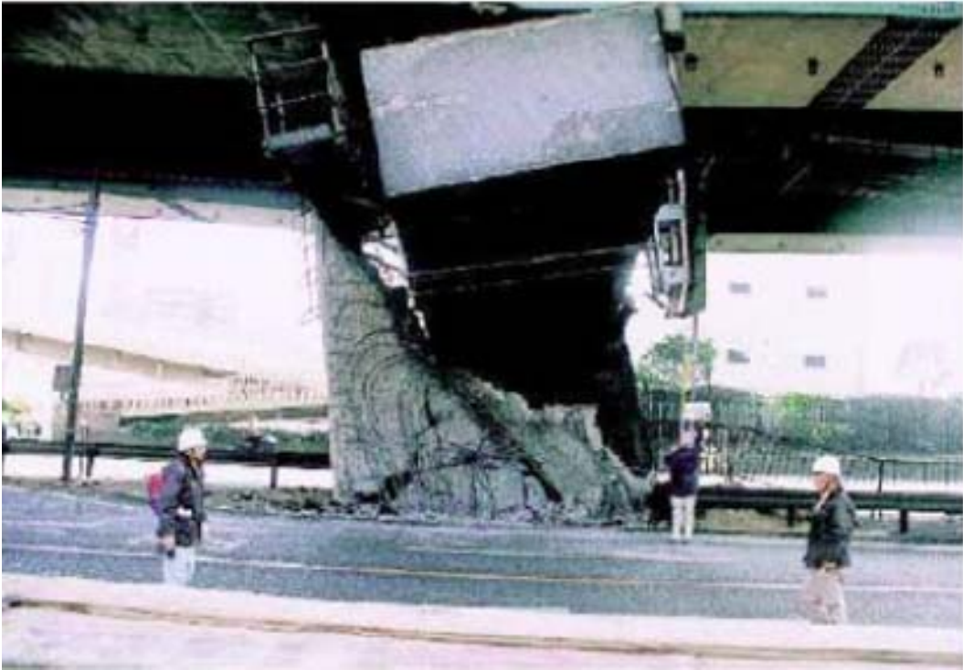
FIGURE 30.51 Shear failure of Pier 150 on Kobe Route 3.
